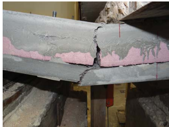
Main Failure Crack
