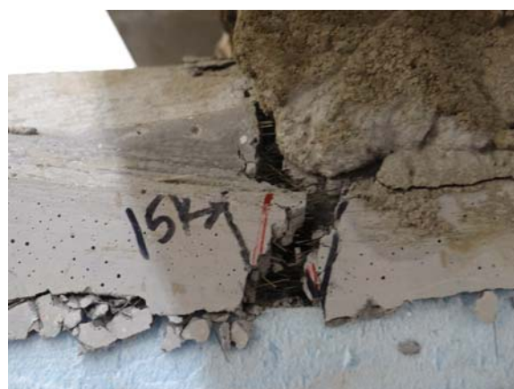
Main Failure Crack
