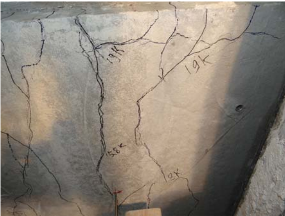
Cracking at Loads
