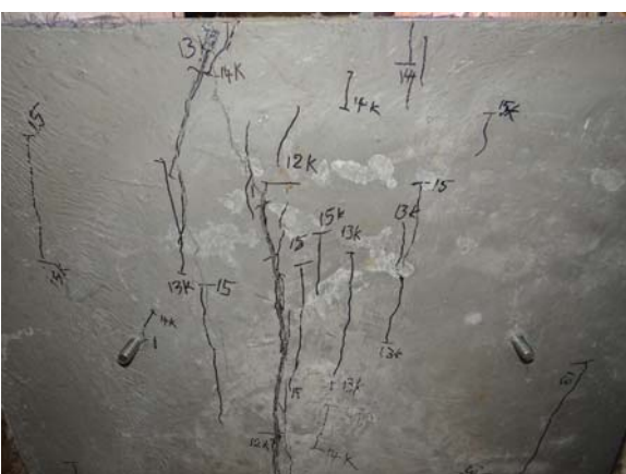
Cracking at Loads
