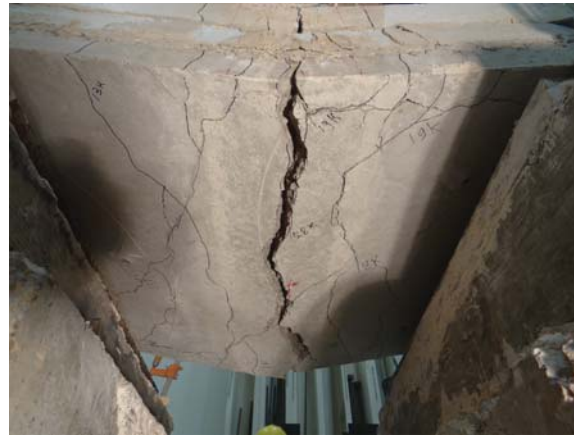
Main Failure Crack
