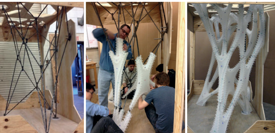
Fig. 10: Plastic formwork assembly process: Assembled steel frame, plastic formwork being tied around steel frame, and fully assembled plastic formwork. (Photo: Brad Bell)
